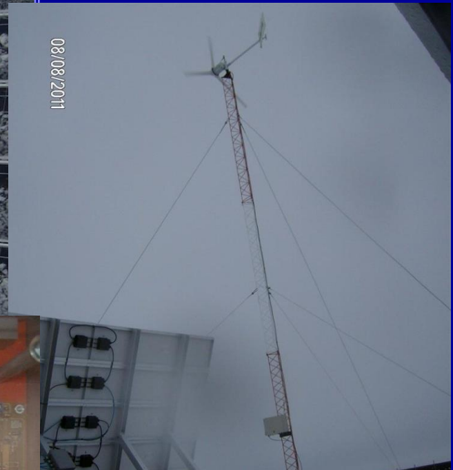
Data transmission for SCADA surveillance
